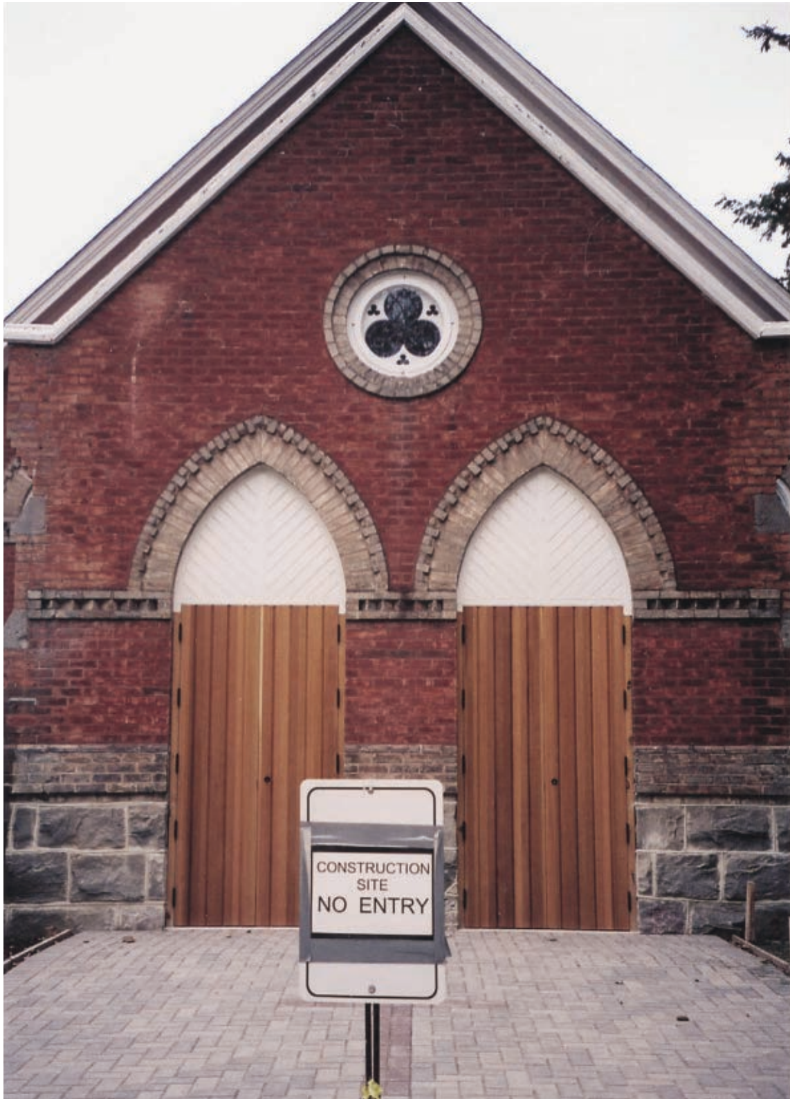
Despite the sign, 150-year-old Heritage United Church in Markham, Ont. still welcomed worshippers during its renovation
